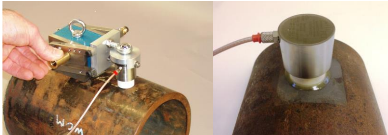
Left: The installation tool for straight pipes (Mag-ST) and a Wi-Corr ultrasonic sensor bonded to a straight pipe section.
